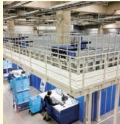
"AutoStore" robotic storage system.
